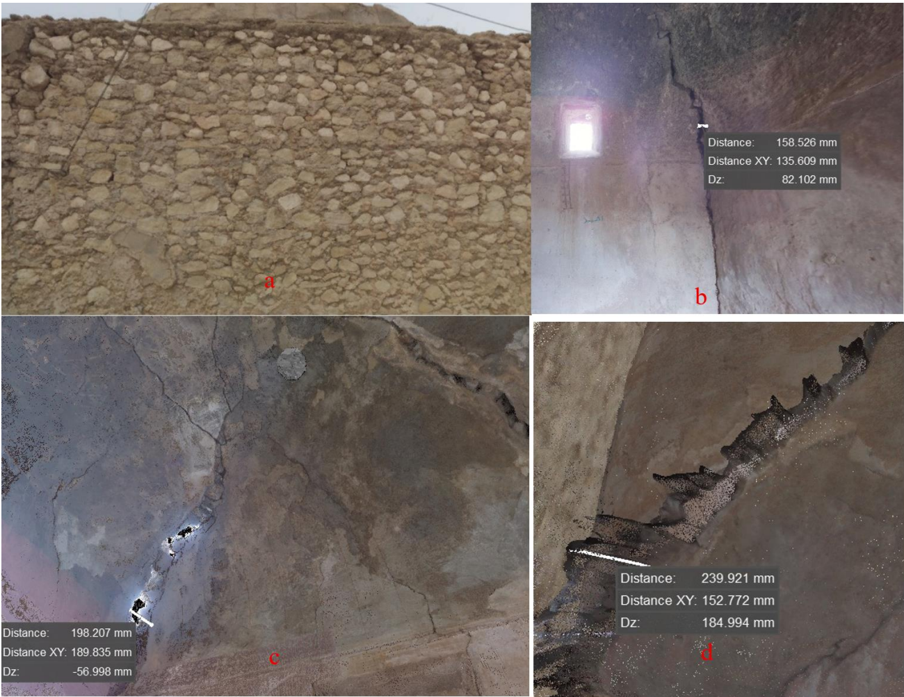
Figure 7: Crack detection and measurements on the non-collapsed part: a) Outside cracks on the wall, b) a crack in the first floor, c) cracks in the second-floor ceiling that have completely made a hole in the ceiling, and d) the depth of the crack on the second.
